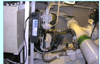
The TRANSMED seawater circuit aboard the M/V Marfret Niolon
